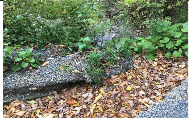
Photo 2: The runoff is eroding a conveyance to the adjacent stream.
