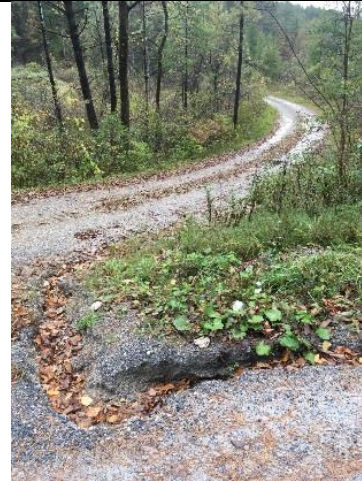
Photo 2: Erosion of Airport Road and the adjacent driveway.
