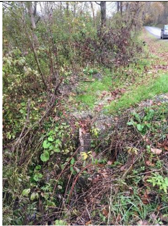
Photo 1: Eroding ditch and conveyance.
