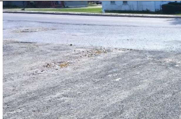
Photo 2: Particulates from the gravel drive flowing to the dry well (top left) may reduce its function.
