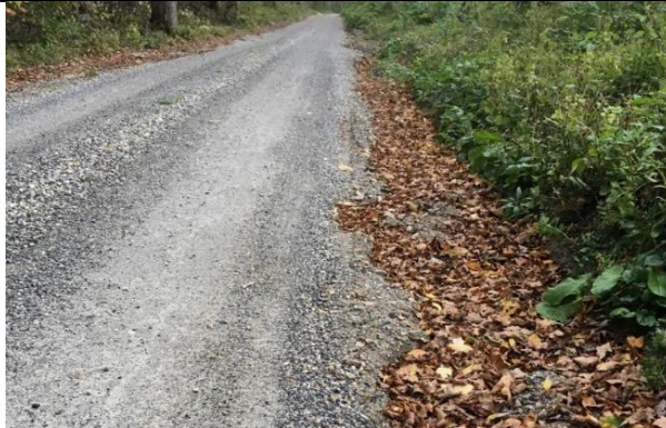
Photo 1: Runoff flowing down Potter Montgomery Road is causing severe erosion of the roadway.
