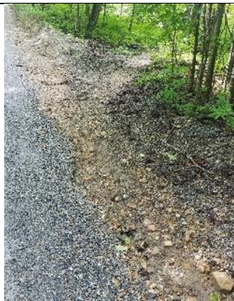
Photo 1: An unstable turnout on the south side of the road.
