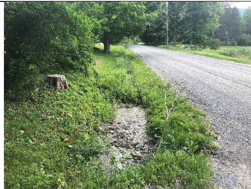
Photo 2: Eroded materials accumulating in the ditch at the intersection of Daniels Road and Glastenview Road.
