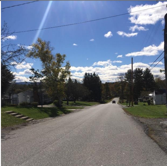
Photo 1: Twitchell Hill Road, with paved ditches draining the left side of the road.
