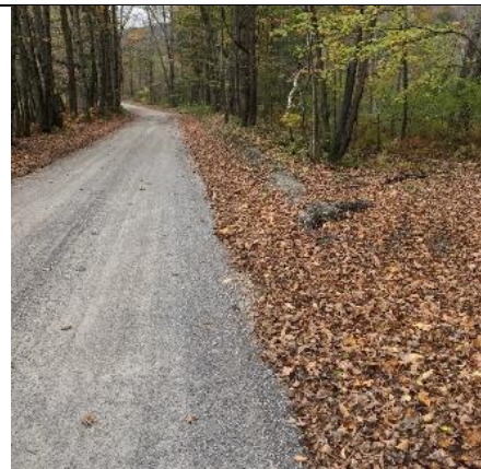
Photo 2: Section of Cross Hill Road without ditches or a stable turnout.
