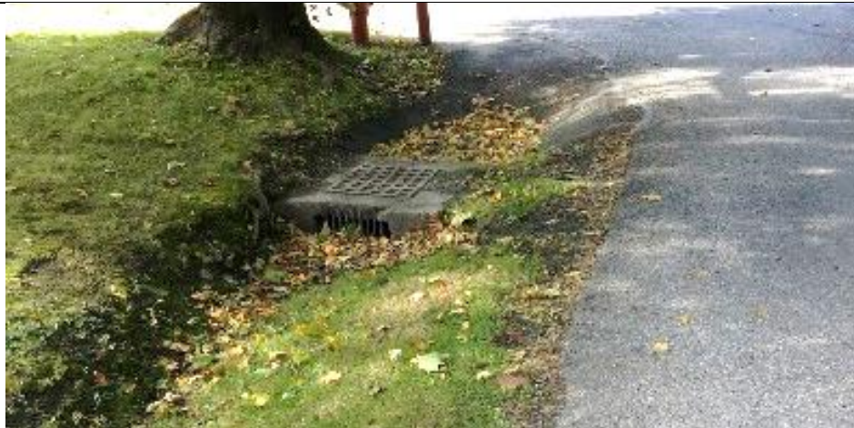
Photo 1: Beginning of the storm drain network at the intersection of Hawks Avenue and Bank Street
