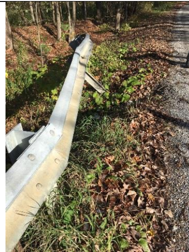
Photo 2: Runoff concentrates along Granger Hollow Road, eroding the area near the guardrail.
