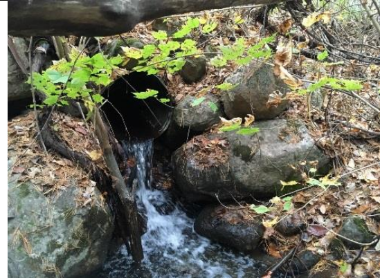
Photo 2: Perched culvert outlet.
