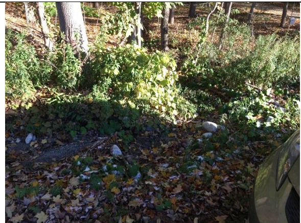
Photo 2: Eroded channel down to stream.
