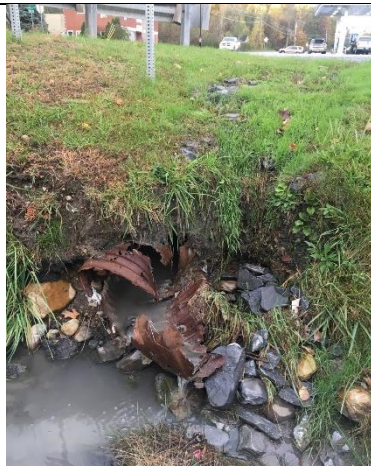
Photo 1: Collapsed stormwater infrastructure outfall with silty runoff from connected impervious.
