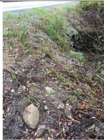
Photo 2: Eroding culvert header and conveyance at the stream crossing.
