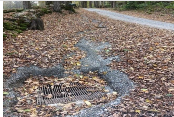
Photo 2: Water flows down the roadway to a driveway culvert with a grated inlet that requires frequent unclogging.
