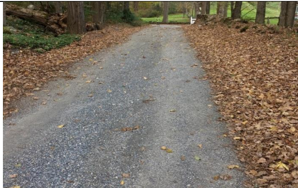
Photo 1: A stretch of Jack Cross Road with no ditches.
