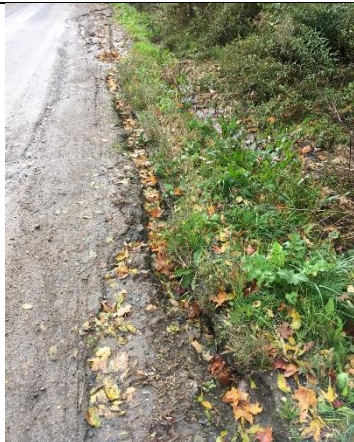
Photo 1: Formation of a secondary ditch due to a grader berm on the north side of the road.
