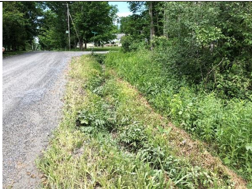
Photo 1: Eroded ditch along Daniels Road.
