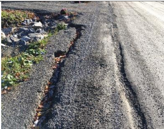
Photo 1: Rilling along road edge.
