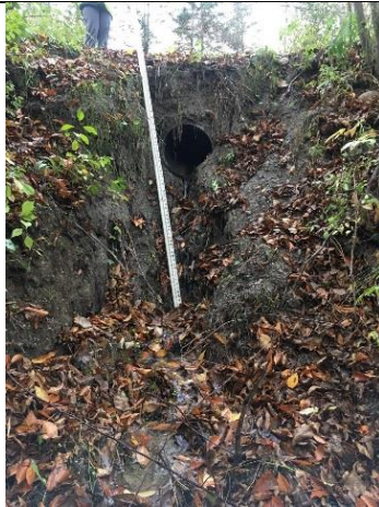
Photo 1: Severe erosion at the culvert outlet.
