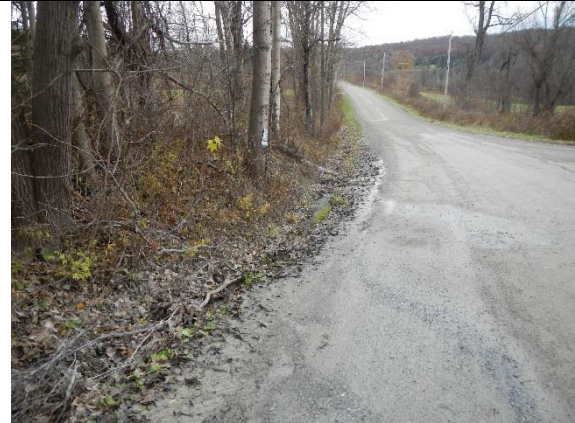
Photo 2: Unstable ditches along Murphy Hill Road.
