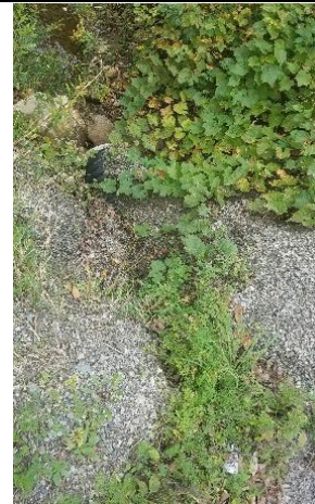
Photo 2: Erosion extends to the drainage culvert.
