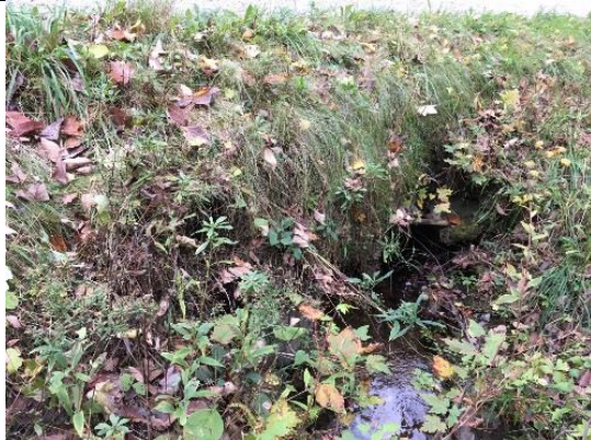
Photo 1: Erosion at the upstream culvert header.
