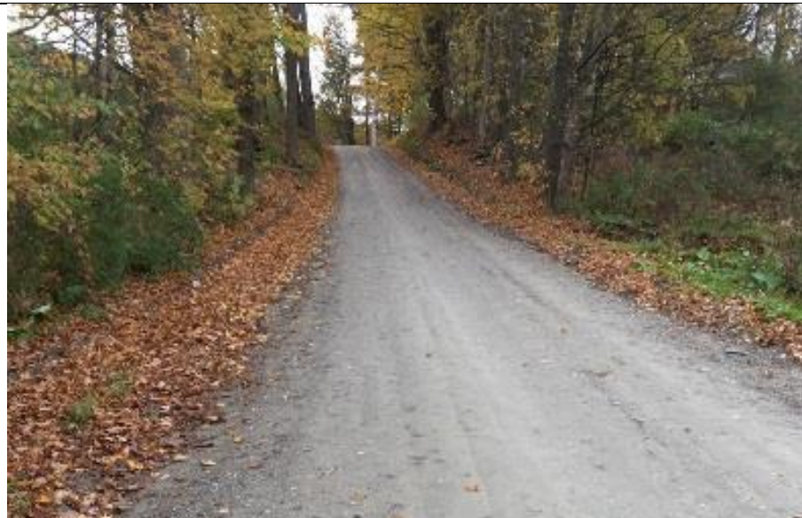
Photo 1: Unstable ditches along Cold Spring Road west of the stream crossing.
