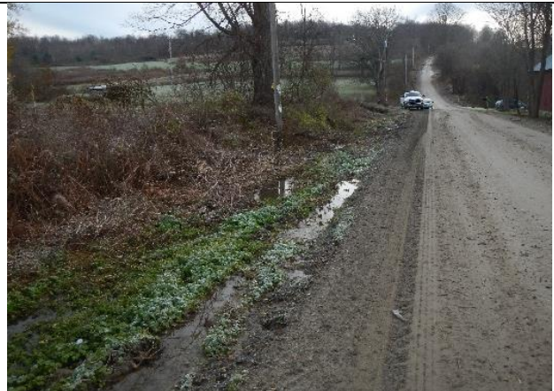
Photo 2: Water pools on the roadway, partially due to runoff from tile drains that are piped into the ditch.
