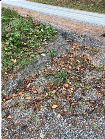
Photo 1: Erosion of the driveway due to concentrated flow from Airport Road.
