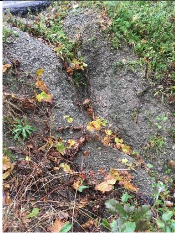
Photo 1: Eroded road embankment.
