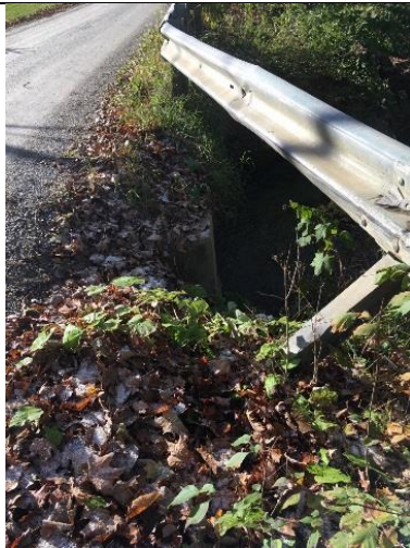
Photo 1: Eroded embankment at the Little White Creek crossing.
